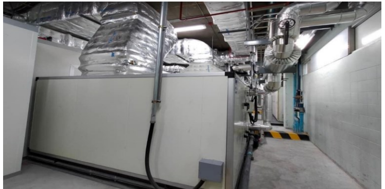
HVAC System (Heating, Ventilation, and Air Conditioning)
